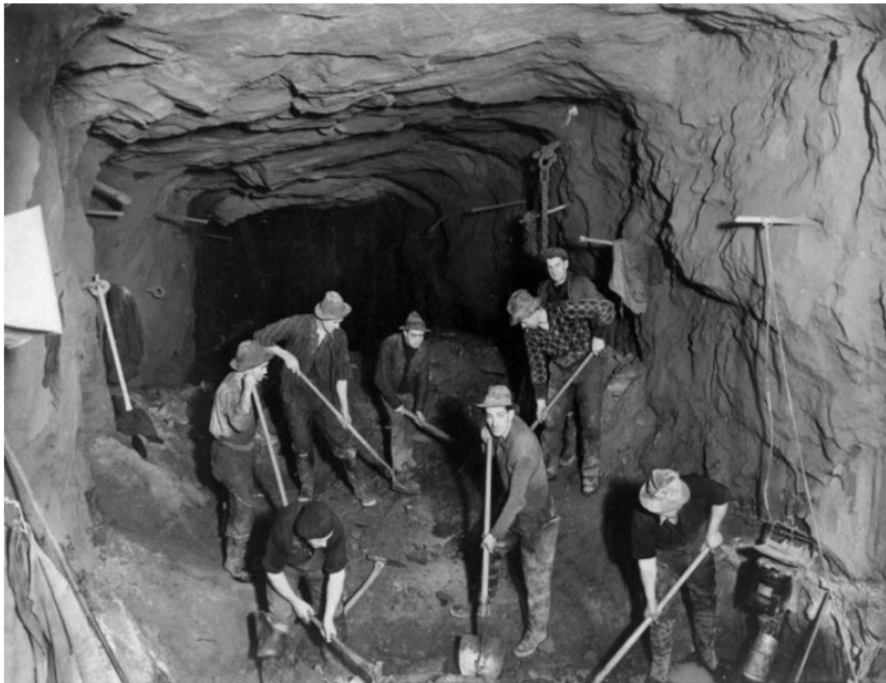
Men at work on the Homer Tunnel, Southland. Raine, William Hall, 1892-1955 :Negatives of New Zealand towns and scenery, and Fiji. Ref: 1/2-024836-F. Alexander Turnbull Library, Wellington, New Zealand. http://beta.natlib.govt.nz/records/22346543
