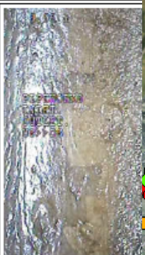
Cracking Circumferential, Large, from 12 to 12 o'clock, (CC LARGE).
